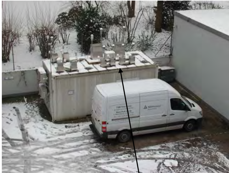
Figure 9: Measuring systems APM-2 on measurement cabinet
