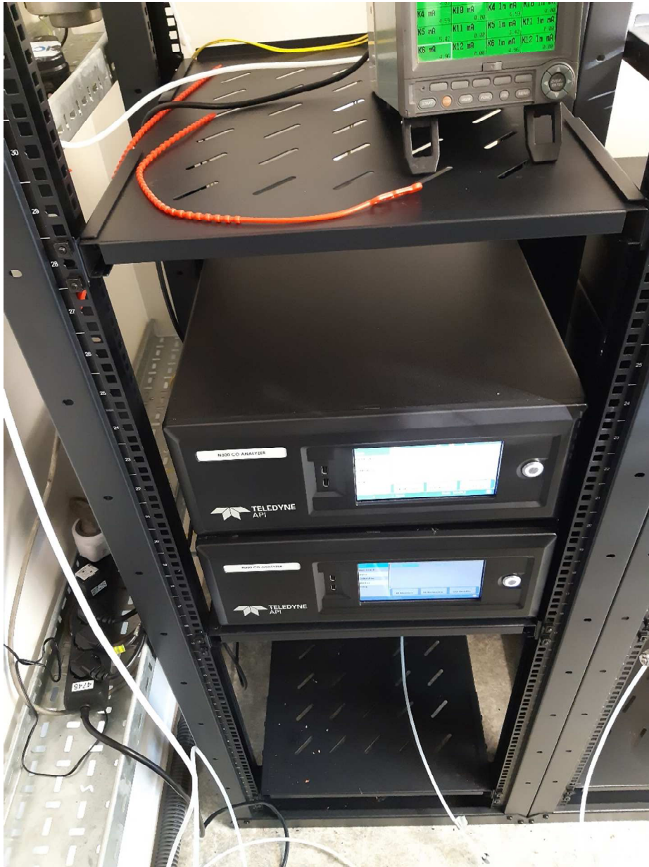
Figure 10: N300 in the measuring station during the field test
