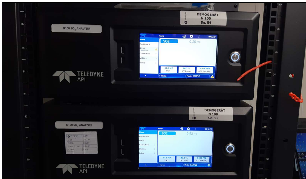
Figure 9: N100 in the measuring station during the field test
